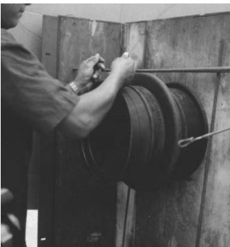
5. For additional stability, it's necessary to secure the sleeve with wire to the rebar. Inset the other end cap firmly and check that second end cap is positioned correctly and close the form.
